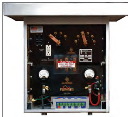
RM4150 Placed in Rectifier
