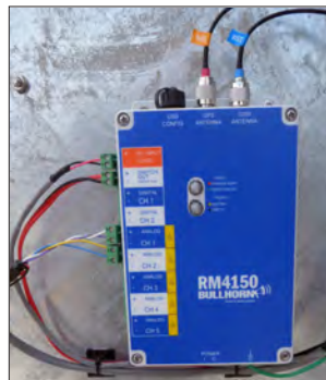
RM4150 Mounted to Rectifier Door
